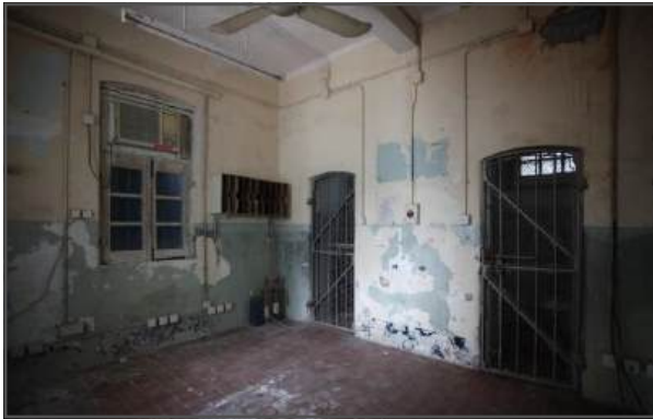
Fig. 9.5 The former Tai O Police Station was in poor condition before revitalisation work began
