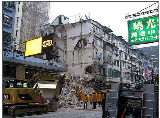
Fig. 2.2 Collapsed building on Ma Tau Wai Road (Source: Baycrest - Wikipedia user - CC-BY-SA-2.5)
