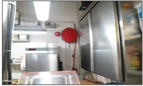
Fig. 7.5 Fire hose reel
